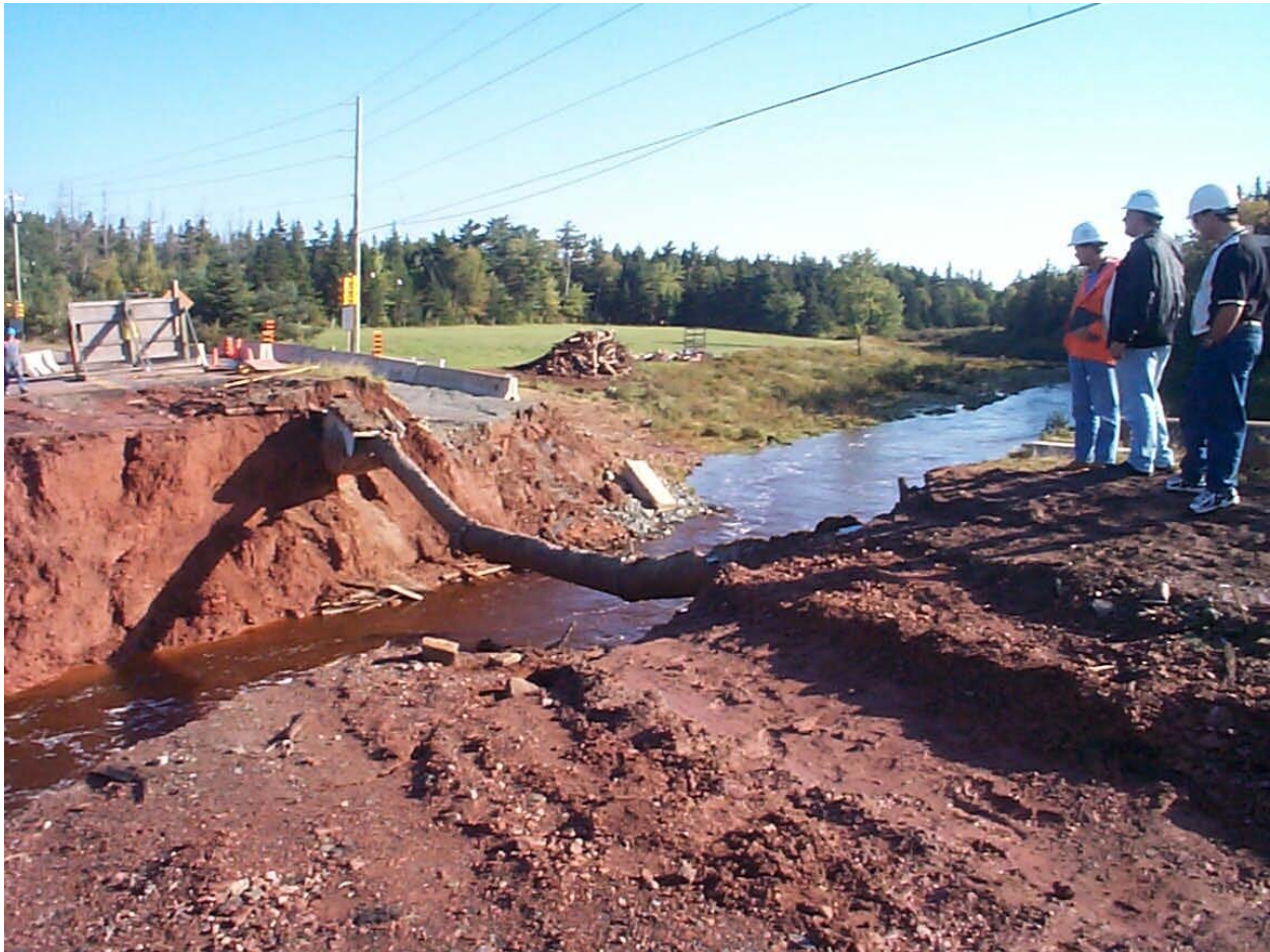
Figure 1: September 1999 storm destroyed a large culvert and severed Amherst's wellfield connection.
