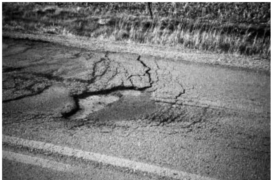
► Loss of bond between pavement layers allows traffic to break loose pieces of surface.
