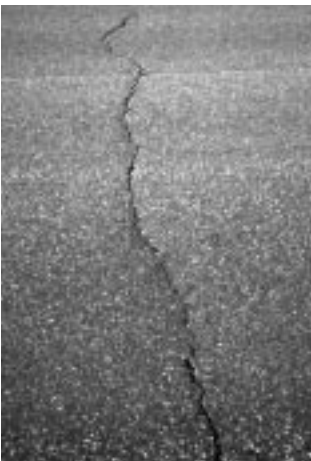
▲ Tight cracks less than 1/4" in width.
