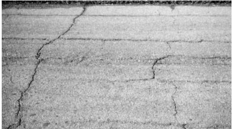
▼ Block cracking with open cracks.
